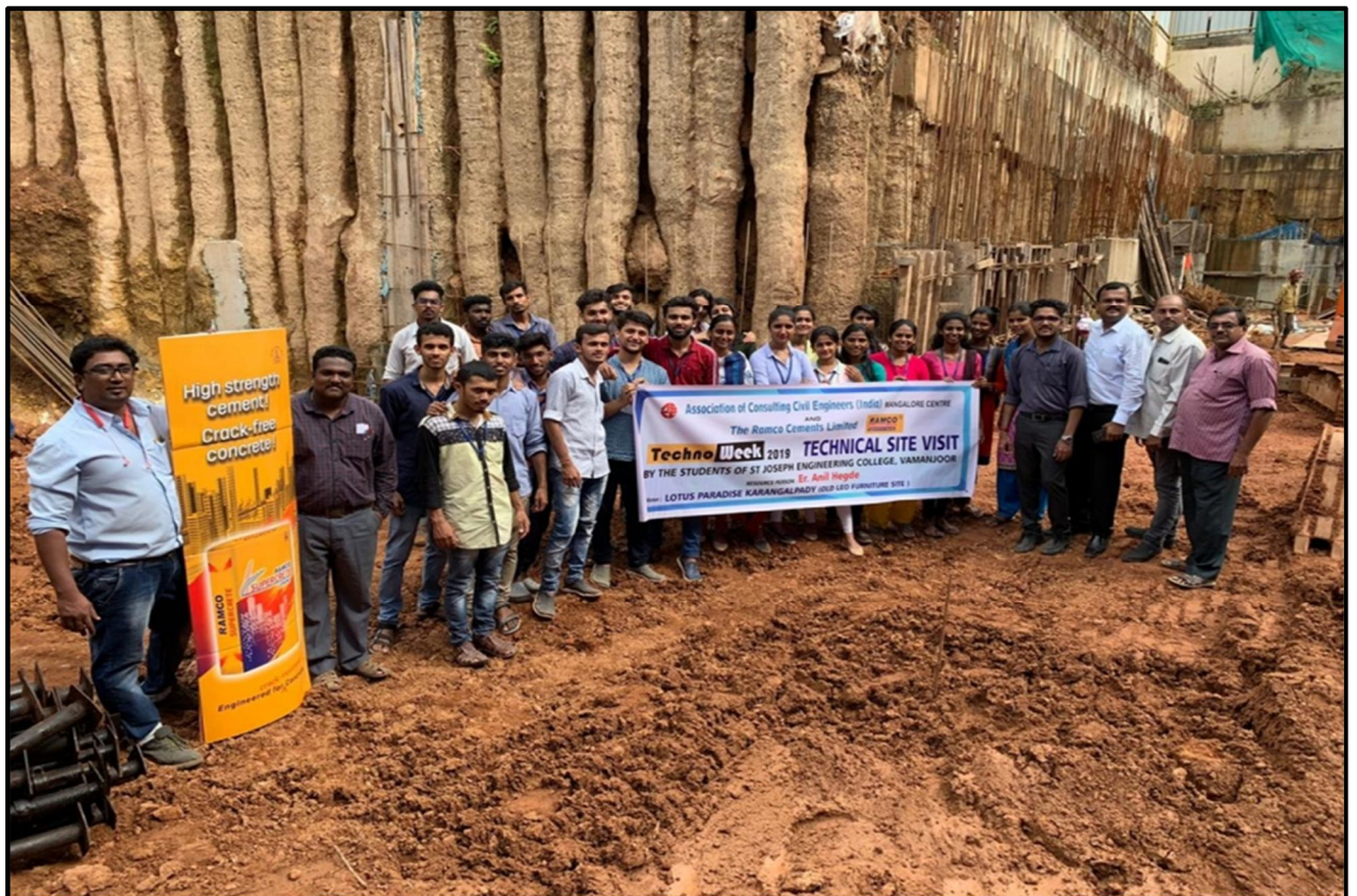
Fig. 26: Industrial Visit to Skyline Signature and Marian Park for Fifth Semester Civil Engineering students, on 24 September 2019, by the Department of Civil Engineering
